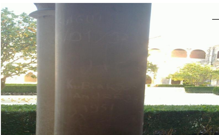
Fig. 39: The Picture of vandalized Column at the Cloister of Dinis
